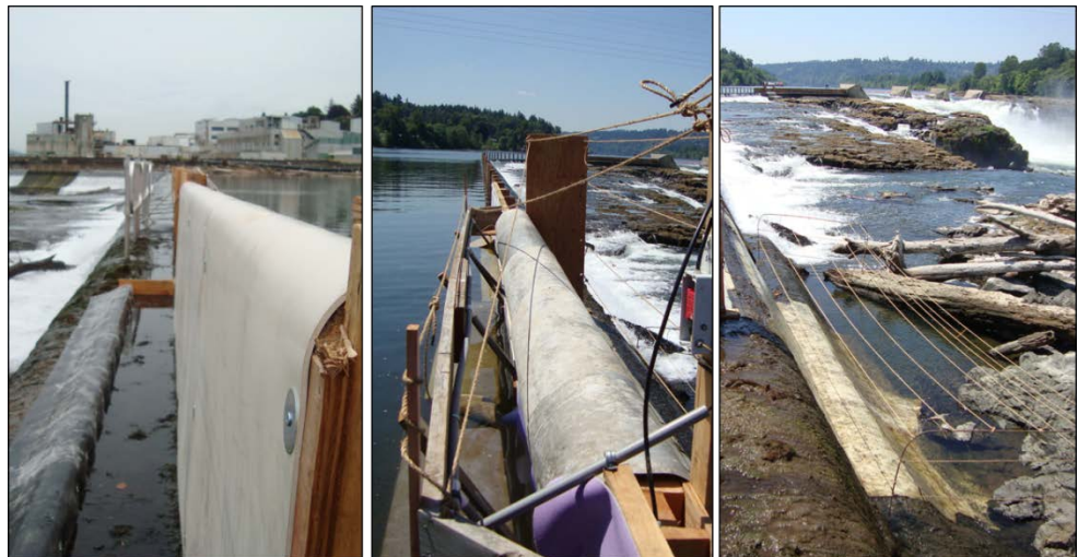
Figure 2. Rubber faced lamprey ramp and resting pool curb (left), debris “cattle guard” (center), and epoxy coated concrete and avian deterrent (right).
